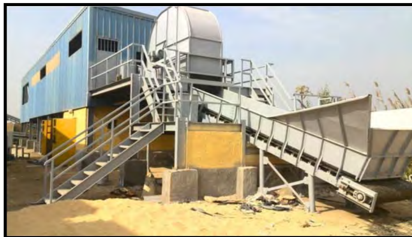
Picture no. (10): Feeding conveyor and bag breaker after rehabilitation process
