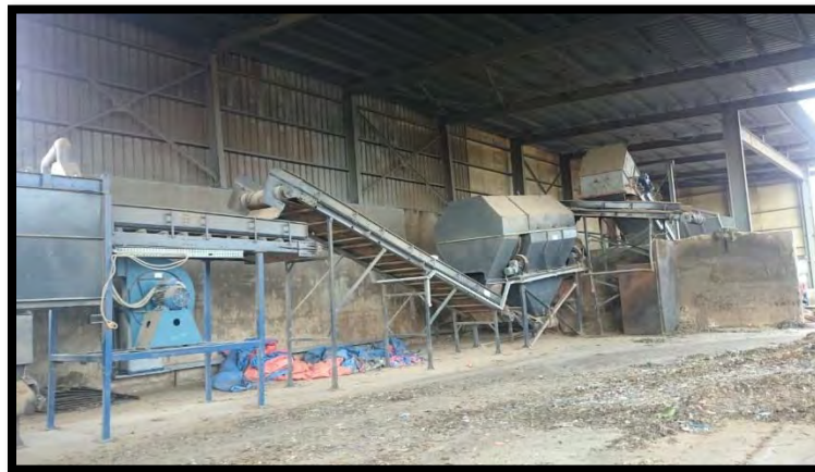
Picture no. (6): RDF Equipment
